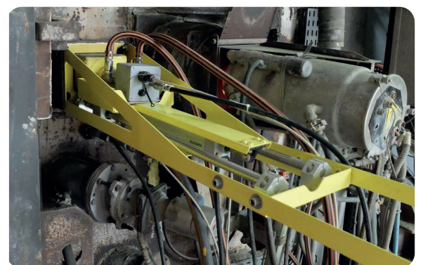
> Pyroscan installed close to the kiln burner
