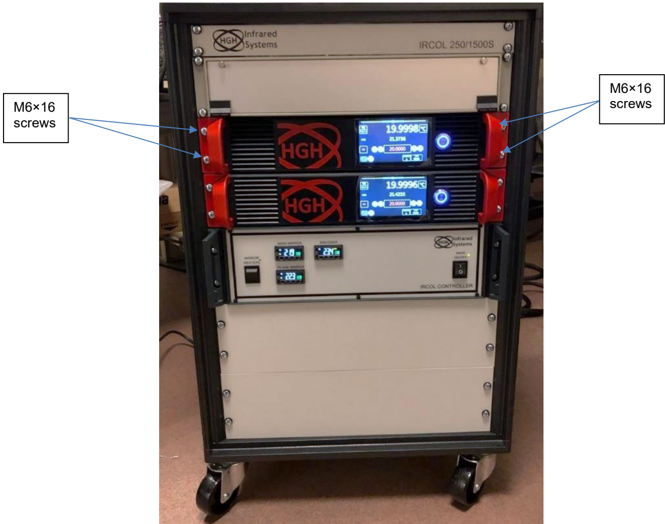
Figure 6: Blackbody controllers integrated inside an electrical cabinet
